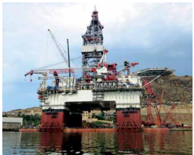
Harnessing the synergies of Keppel O&M's global resources, including support from a team of 80 from Keppel FELS, work on the first modern semi to be completely built in Azerbaijan is in an advanced stage
